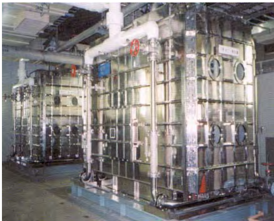
T11 Advanced treatment plant in Kanamachi
