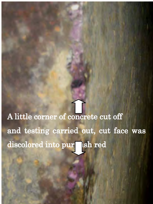
Picture Phenol-Phthalein Testing on the wall of utility conduit of Pulsator at WTP No.2
