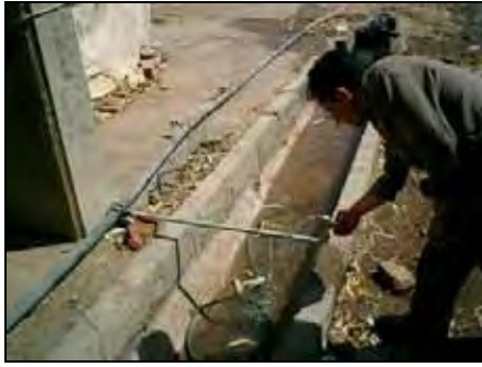
Ground-surface piping and temporary water taps in Bam City
