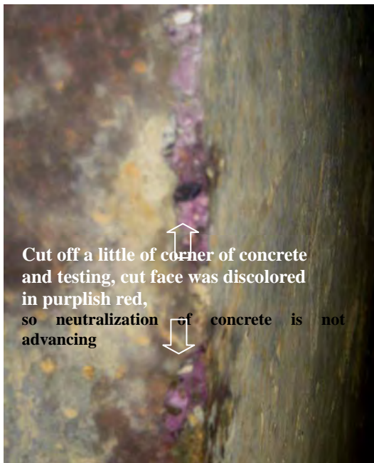
Picture 4.2.7 Phenol-Phthalein Test on the wall of utility conduit of Pulsator at WTP No.2
