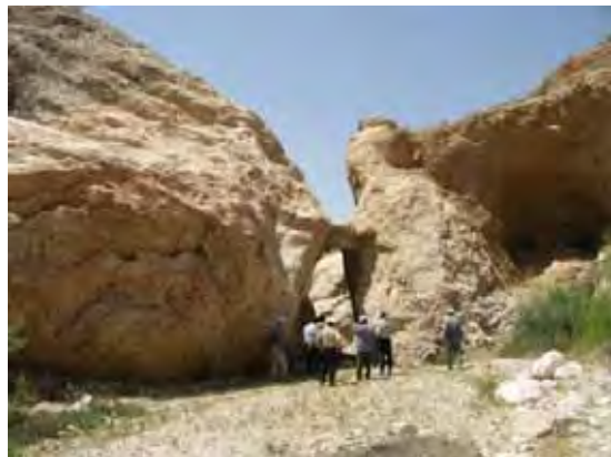
Breached Upper Sabo Dam
