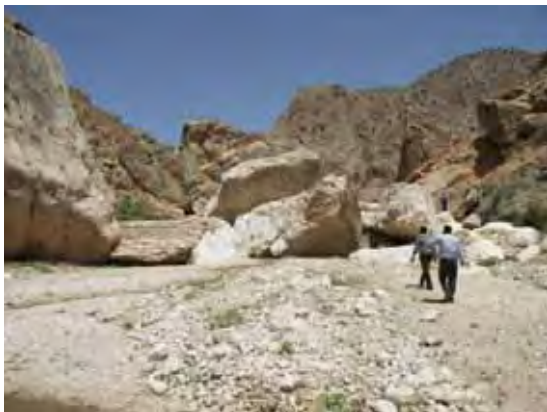
Broken Intake Structure
