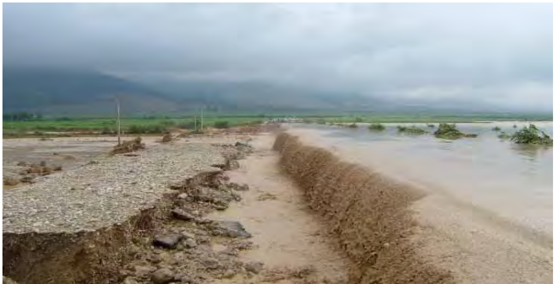
Overtopping the Gorgan-Mashhad Road
