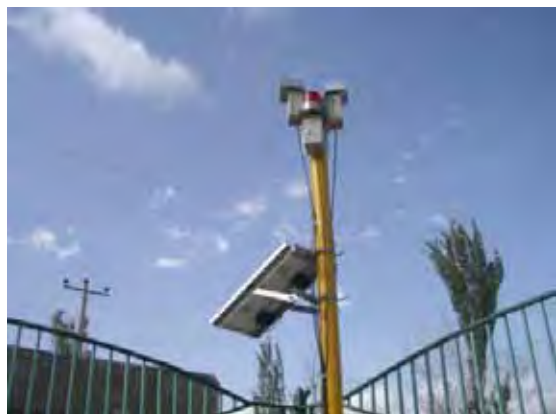
Emergency Equipment installed by the JICA Study Team
