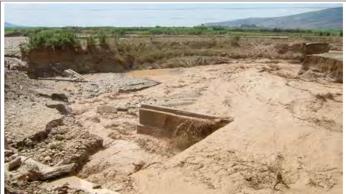
Floodwater through the 14 Metry Bridge
