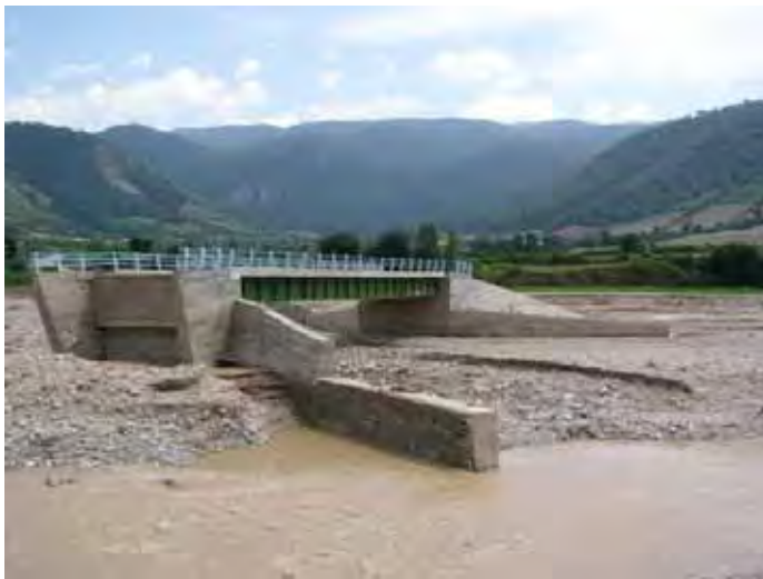
Both sides of approach were washed away.
