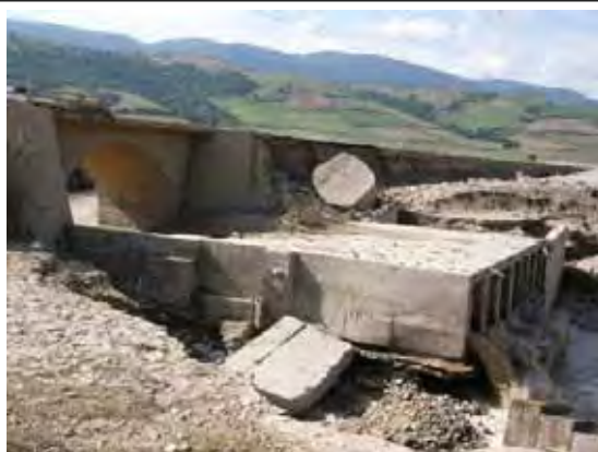
Damage on the 14 Metry Bridge
