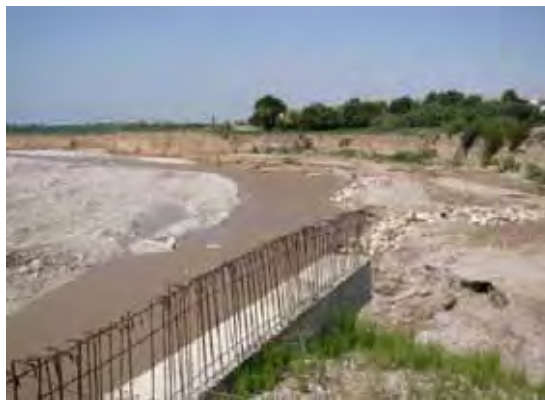
After the 2005 Flood, Washing out Spur Dike
