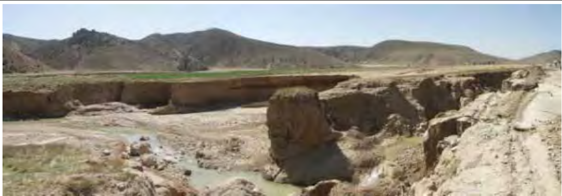
After the 2005 Flood. Erosion was progressed upwards in 30 to 50 m by the 2005 Flood.
