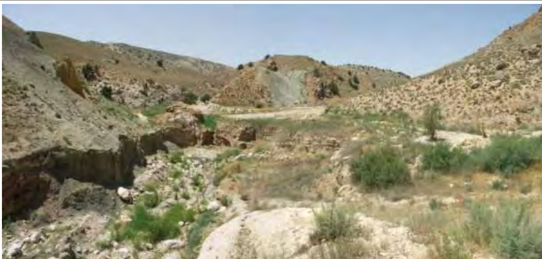
Sediment Accumulated in the Upper Basin of the Upper Sabo Dam viewing from the Dam Embankment
