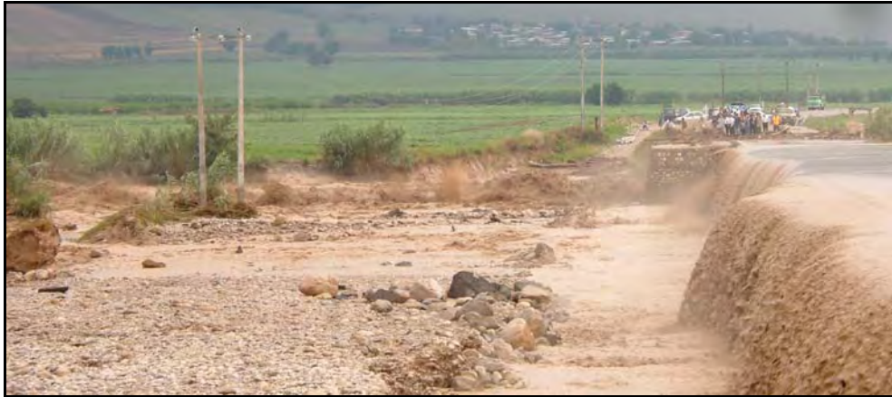
Figure 6.6: Backwater at 14 Metry Bridge, photo from 10 August 2005.
