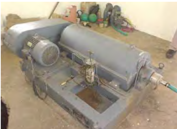
Sludge treatment facilities Centrifugal dewatering
