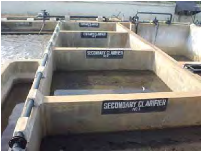
Treatment facility. Secondary clarifier and tertiary clarifier
