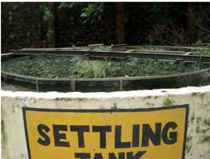
Secondary sedimentation tank covered with thick scums and some plants
