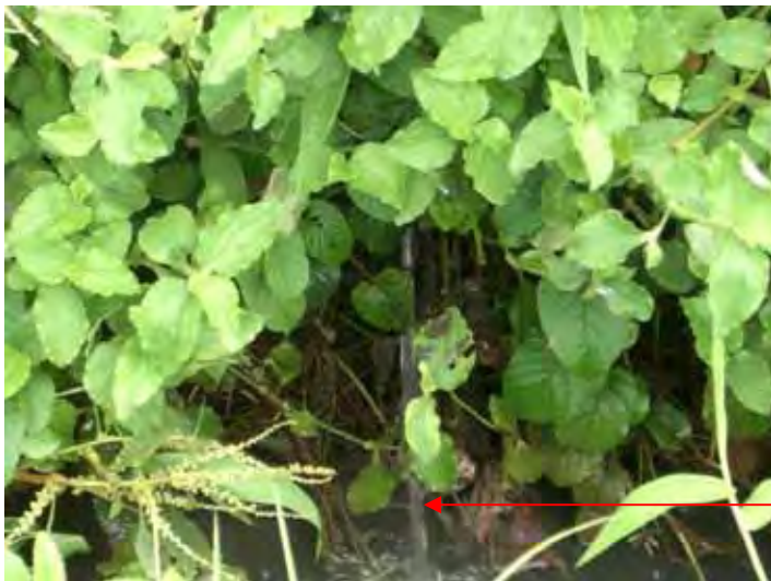
Discharging point of overflow effluent from soak pit into a side ditch of road
