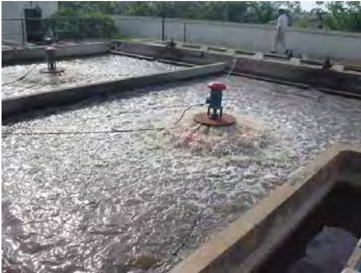
Treatment facility. Aeration Tank
