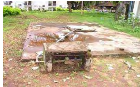
Underground closed water tank having metered water connection in a hotel
