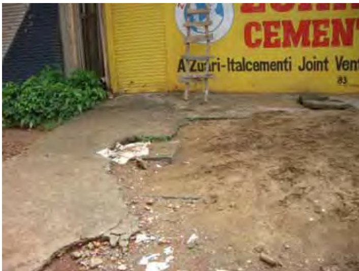
Top of Septic tank and soak pit, covered by concrete slab and pavement
