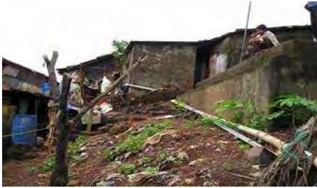
Home wastewater pipeline and septic tank in Monte Hill, Margao
