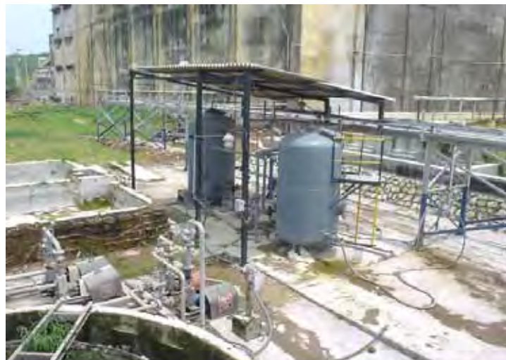
Sand filtration tank for treated water of secondary treatment facility
