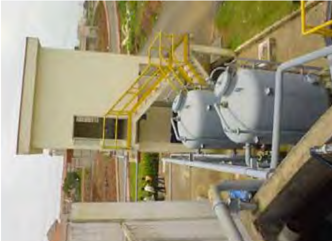
Treatment facilities Sand filtration tank
