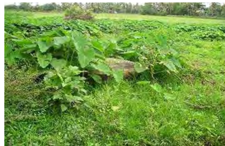
Sewerage manhole chambers overflowing in wet season in Margao
