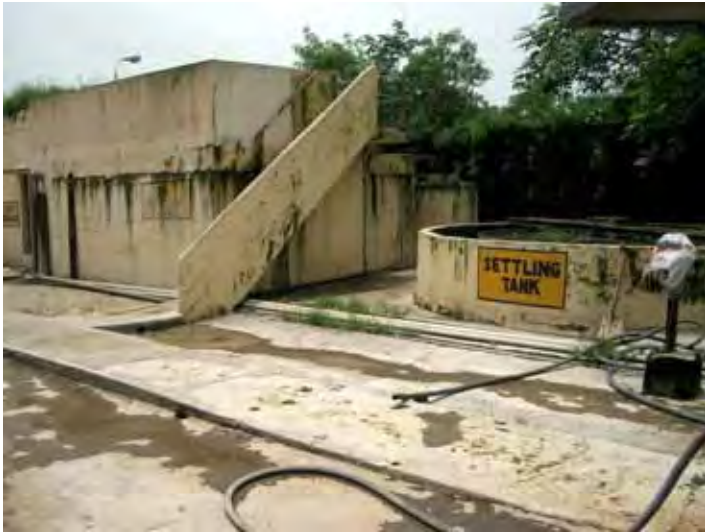
Treatment facility for domestic wastewater of employees. Aeration tank and secondary sedimentation tank
