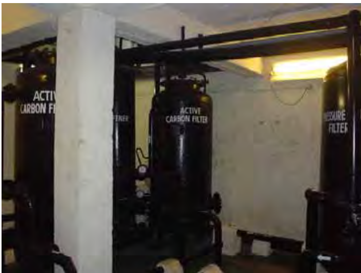
Treatment facility. Activated carbon adsorber
