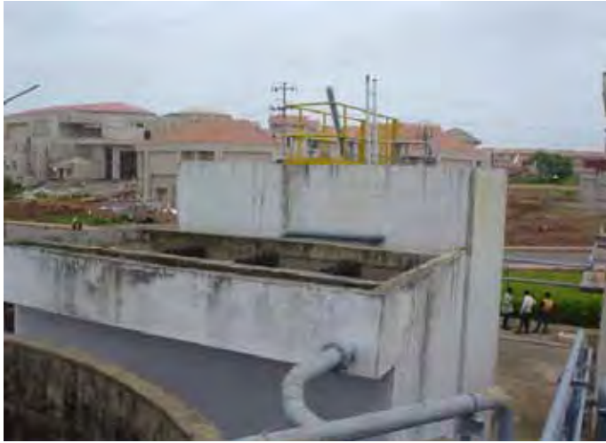
Treatment facilities Aeration tank and secondary clarifier
