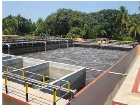
Photo 32.4 SBR Reactor Tank
