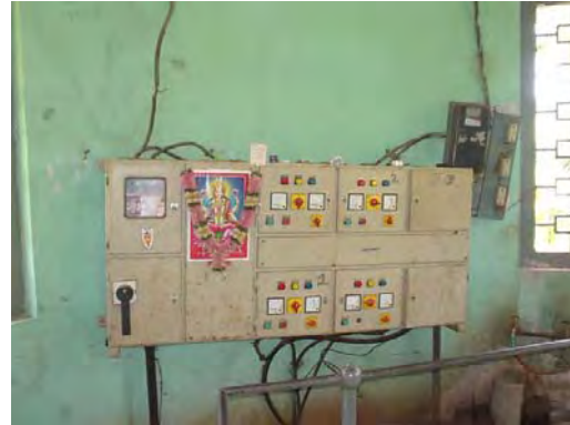
Photo 32.10 Deteriorated Electrical Panel
