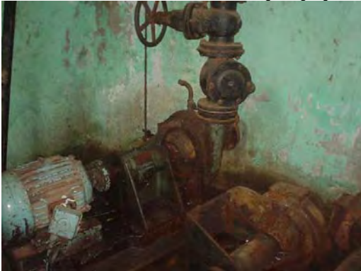
Photo 32.9 Deteriorated Pump Equipment
