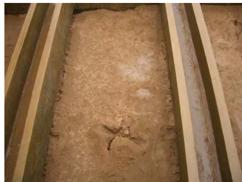
Photo 31.10 Filter Media of Podocem Plant
