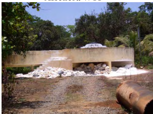
Photo 31.11 Chemical Storage at the Assonora WTP
