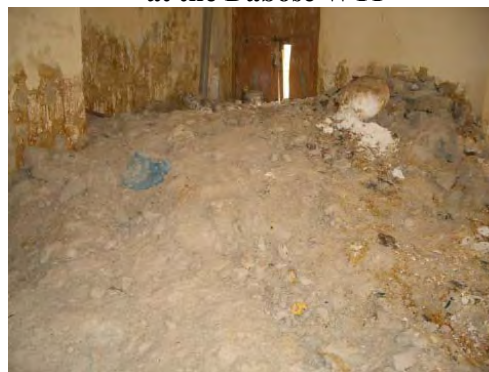
Photo 31.12 Chemical Storage Room at the Dabose WTP
