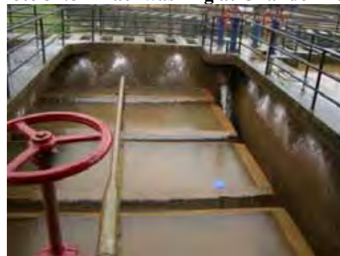
Photo 31.8 Backwashing at Chandel Plant
