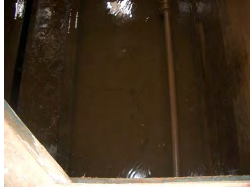
Photo 31.9 Backwashing at Assonora Plant
