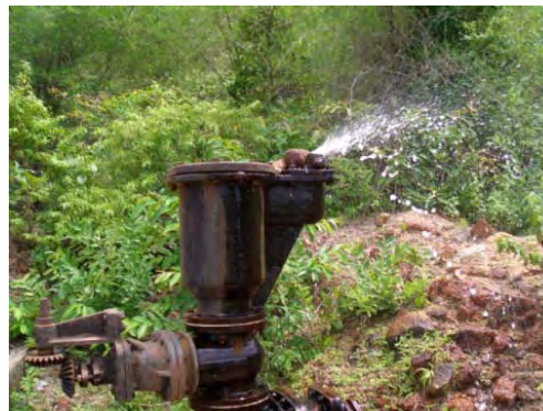
Photo 31.3 Leakage from Air Valve along the Transmission Main
