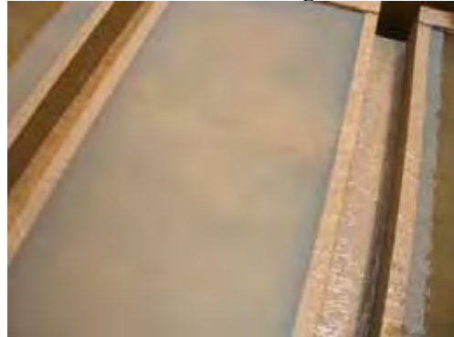
Photo 31.5 Backwashing at Plant IV
