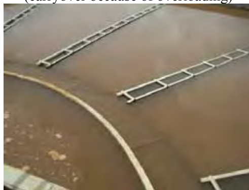
Photo 31.4 Sedimentation Basin at Plant IV (carryover because of overloading)
