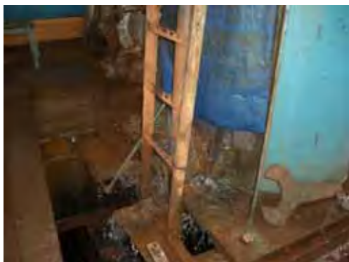
Photo 31.6 Leakage from Intake Pump at the Curti Plant
