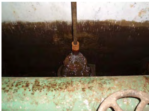
Photo 31.2 Leakage from Valve at Salaulim WTP
