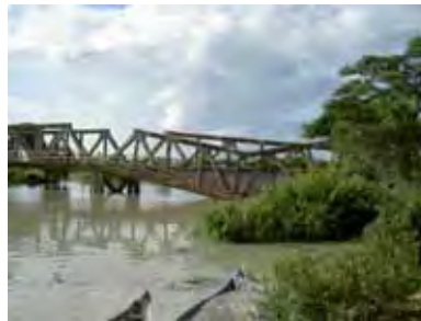
Collapsed Concrete Truss Bridge (NR.6)
