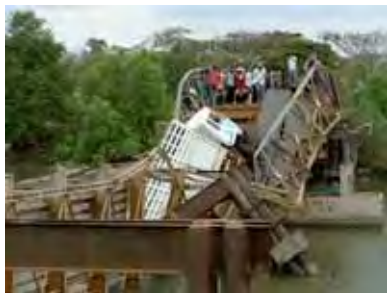
Collapsed Bailey Bridge (NR.33)
