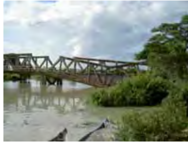
Collapsed Concrete Truss Bridge (NR.6)
