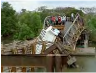
Collapsed Bailey Bridge (NR.33)
