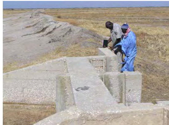
Dike against the salinization (Region of Fatick)
