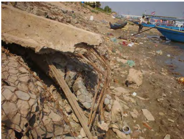
Photo 2.2.2 Collapse in the Old Market East Revetment (1)
