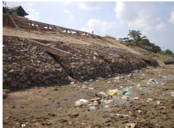
Photo 2.2.3 Collapse in the Old Market East Revetment (2)
