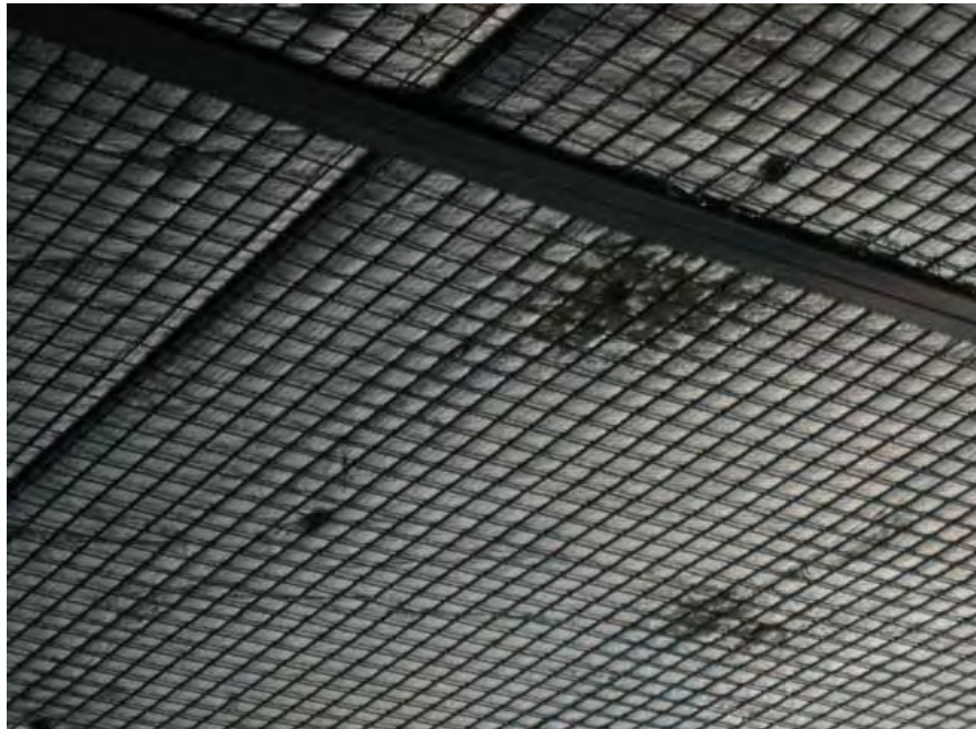
A closer view of the worn out ceiling
