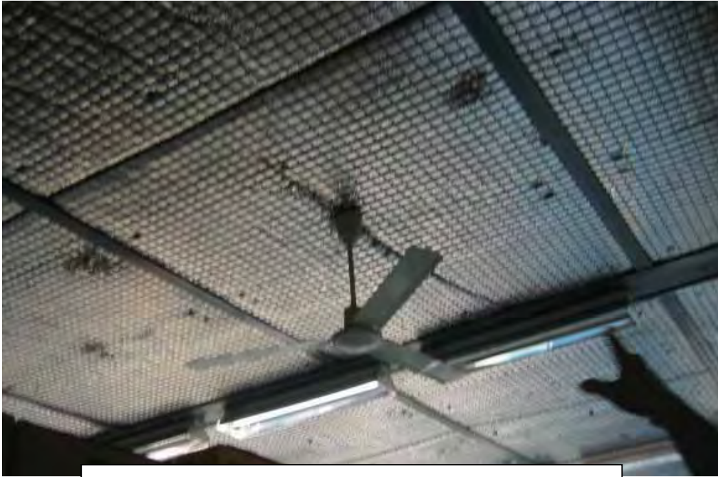
Worn out ceiling of the BPS testing center
