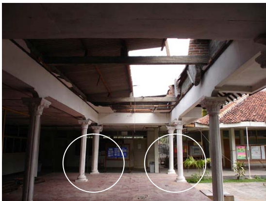
Bantul 2 Secondary School: pillars and beams are not linked, making the structure unstable.
