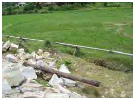
K3-1 Dak Ui JICA 導水管
