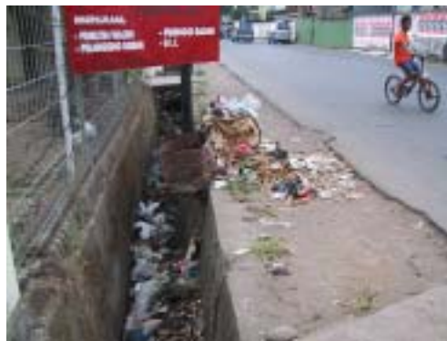
(Stuck drainage canal where solid waste is dumped)
