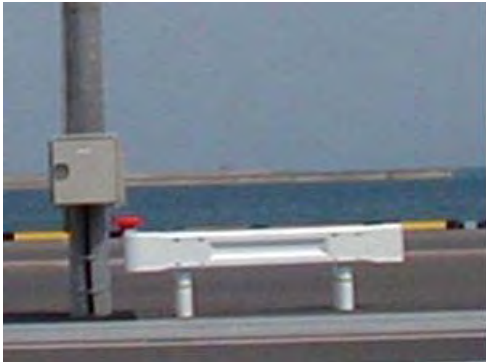
Photo 15-2-5-5 Site Condition of Protector for Security Equipment
