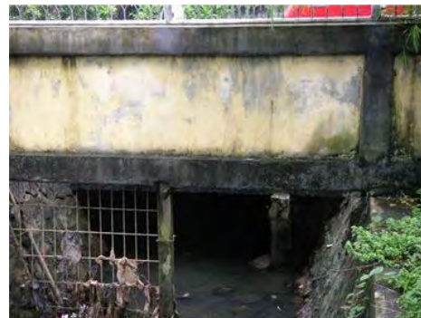
Fence covering left half of drainage (The fence should cover the right half as well.)
