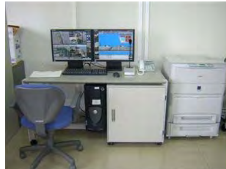
Monitoring room in the port
