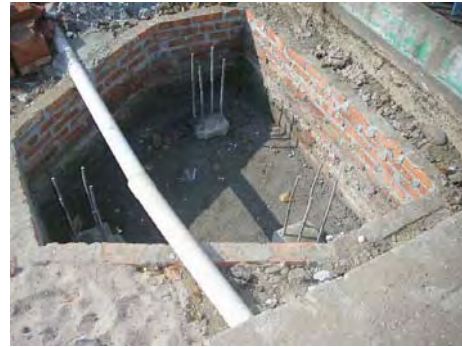
Camera pole base
