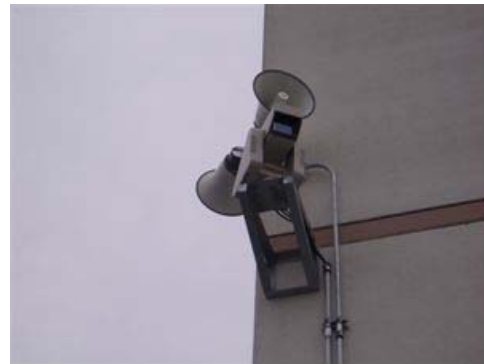
Right → CCTV camera and speakers are on the wall of an administration building. (Speakers are directly fixed on the wall.)
