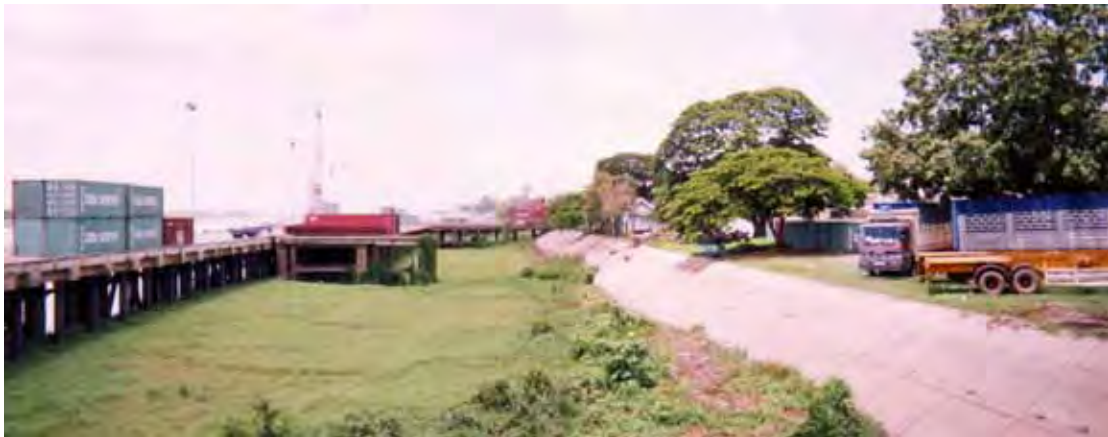
Wharf structure are of the concrete deck supported by point baring piles. Left side is berth area and right side is port yard.
