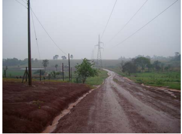
Road condition becomes worse when it rains
