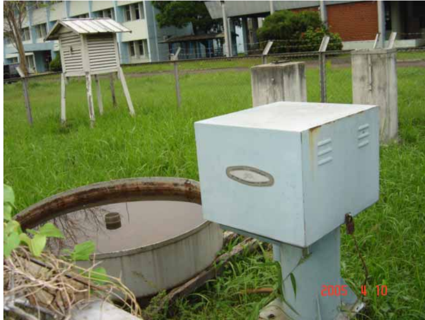
Photograph No. 1. Recording rain gauge and evaporator ERR-101 still functioned well at Irrigation Center, Bekasi
