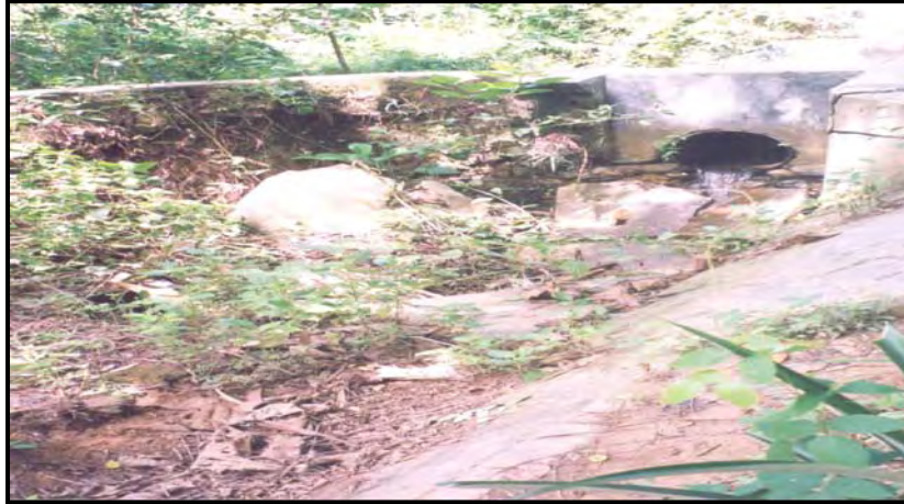
Irrigation canal was damage in Ranomeeto village
