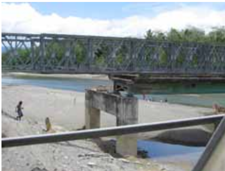
Photo 2.2 Two spans missing of the old bridge
