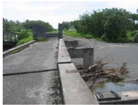
Photo 2.3 Superstructure bended to downstream
