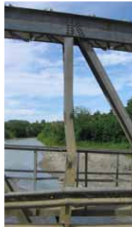
Photo 2.5 Vertical member damaged by hit
