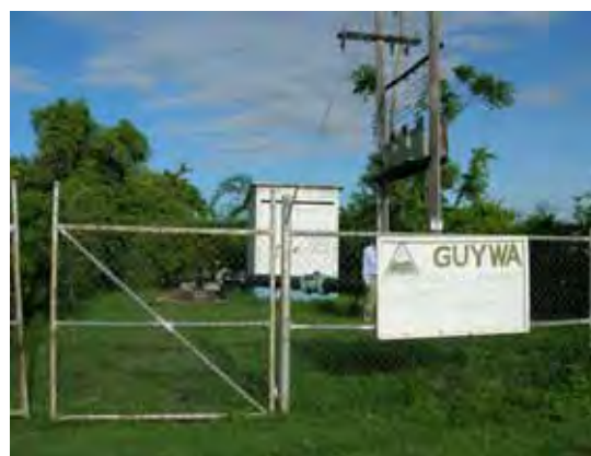
Existing Spring Garden pumping station. This well is a water source of the Queenstown WTP.
