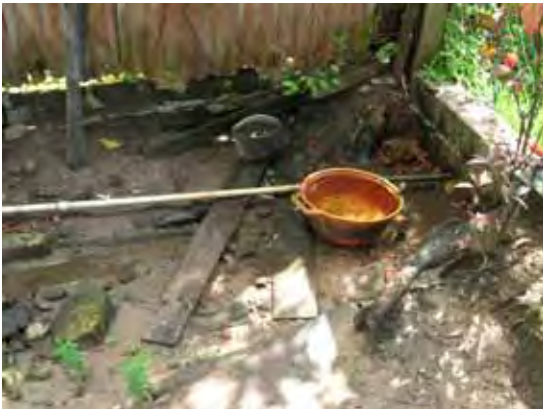
Low pressure water supply. Residents of this house can receive water only from this hydrant set at ground level.
