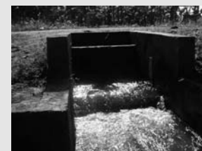
Measuring Device at the Head of F-canal (Control Area, LB Tract 2)
