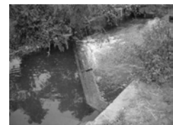
(Above) Duckbill weir in the upstream of FC-9. (Below) Diagonal weir in the upstream of FC-12
