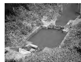
(Above) Neyrpic Automatic Head Control Gate (downstream view) (Below) -do- with baffle distributor
