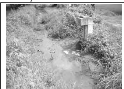
Distributory Canal 1 in LB Tract 2 Sedimentation and Vegetation inside the Canal (Rajangana Major Scheme)
