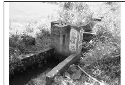
Turnout on D-canal Missing Gate (Nachchaduwa Major Scheme)
