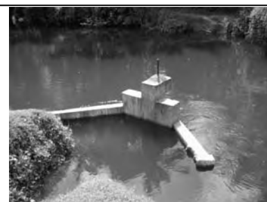
Turnout on Main Canal (Head of D-canal) Submerged due to Excessive Discharge and Canal Slope Erosion (Rajangana Major Scheme)
