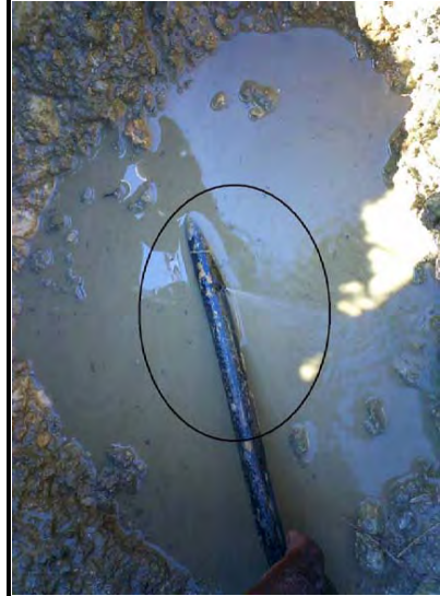
Crack by stone
