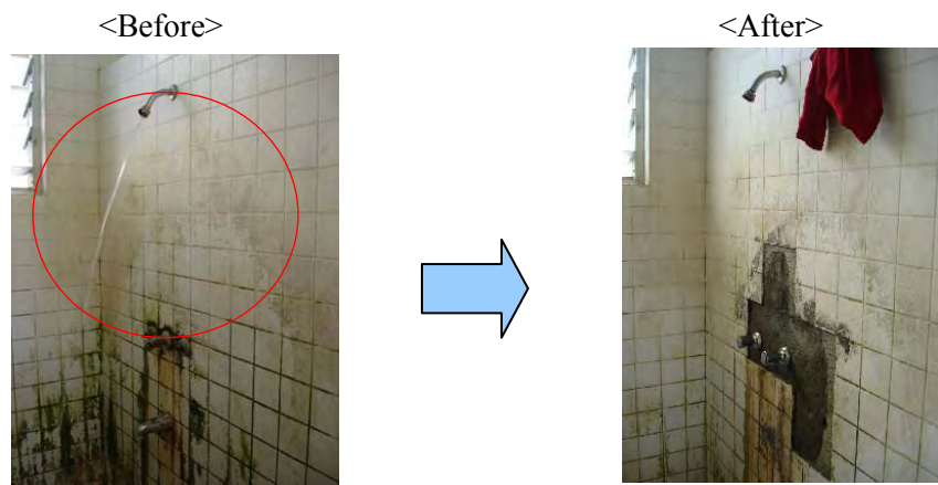
b. Leakage of Shower (at Honiara Hospital)
