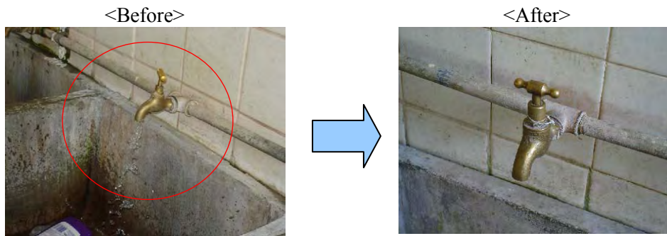
a. Leakage of Wash Basin (at KG VI School)
