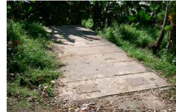
Tuvaruhu Communal Septic Tank
