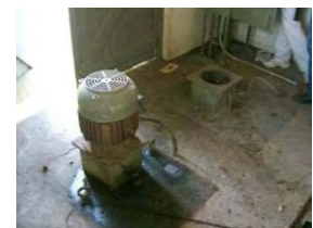
KG VI Pump Station
