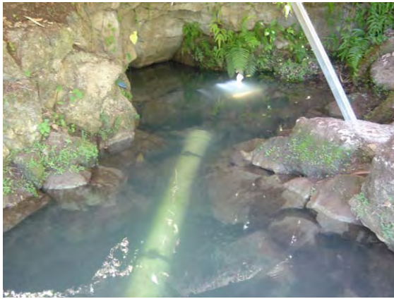
Water intake point of Konglai Spring. This spring is the main water source for Honiara covering 50% of distribution volume. However, the distribution volume is reduced to less than 40% due to the blockage occurred in October 2005.
