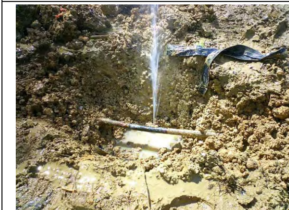
Leakage from water distribution branch pipeline (diameter of 50mm, galvanized iron pipe). Water is being spouted from the pipe.
