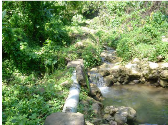
Water conveyance pipe which conveys water from the intake point of Konglai Spring to transmission pump station.
