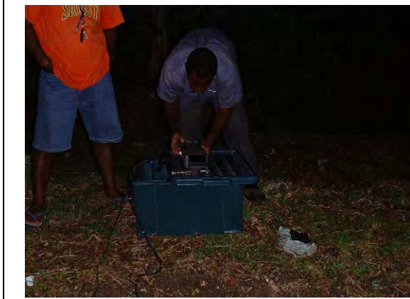
Pilot project for establishing leakage reduction indicator. 12 model sections were selected by the leakage survey. This photo shows the situation of the work at Vavaya Ridge district. Leakage (or minimum night flow) is measured before pipe replacement.
