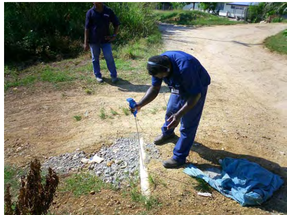
Leakage detection survey done in Phase-1 of this Study SIWA staff is surveying the leakage sound by means of digital sound detector.
