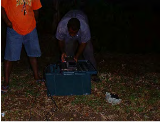
Pilot project for establishing leakage reduction indicator. 12 model sections were selected by the leakage survey. This photo shows the situation of the work at Vavaya Ridge district. Leakage (or minimum night flow) is measured before pipe replacement.
