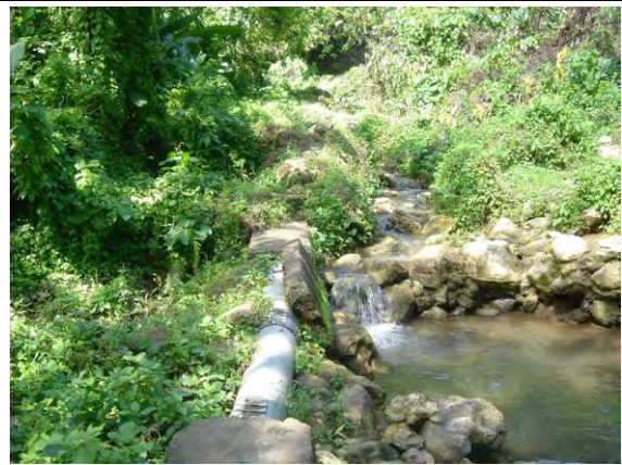
Water conveyance pipe which conveys water from the intake point of Konglai Spring to transmission pump station.
