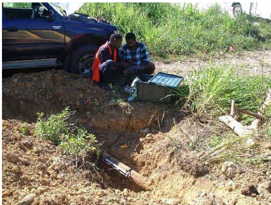
Situation of leakage measurement work before pipe replacement at Kola Ridge district.
