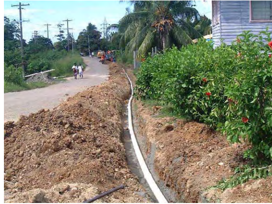
Situation of pipe replacement work at Vavaya Ridge district. About 100m of pipe was replaced in one section.
