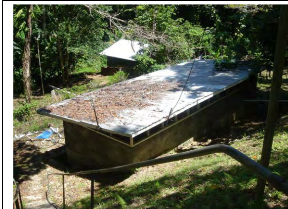
Chlorination injection house located downstream to Rove Spring.
