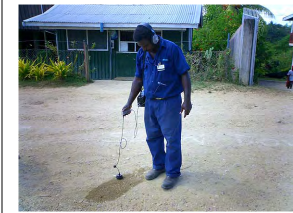
Leakage detection survey done in Phase-1 of this Study SIWA staff is doing the detection survey by means of leakage detector.
