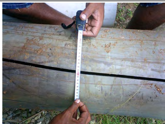
On the water distribution main (diameter of 300mm, PVC pipe), large leakage may occur through large crack on the pipe.
