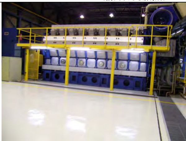
PT. MAKASSAR POWER (発電機)
