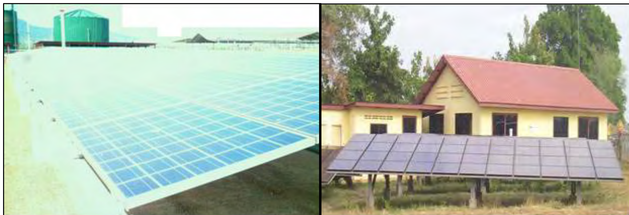
(a) Large scale PV (50 kWp) & biogas hybrid system (b) Large scale PV (30 kWp) & MH hybrid system
