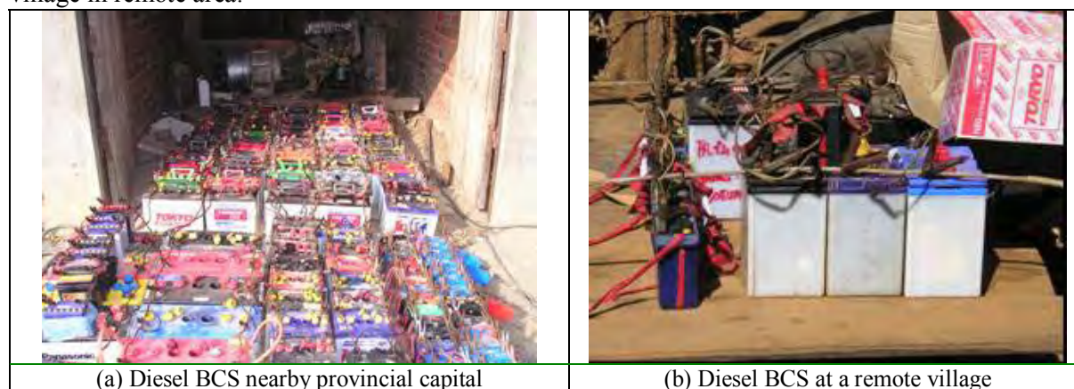
Figure 3.5.1 Typical Diesel BCS
