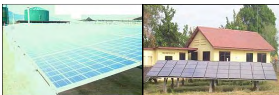
(a) Large scale PV (50kWp) & Biogas Hybrid system (b) Large Scale PV (30kWp) & MH Hybrid system
