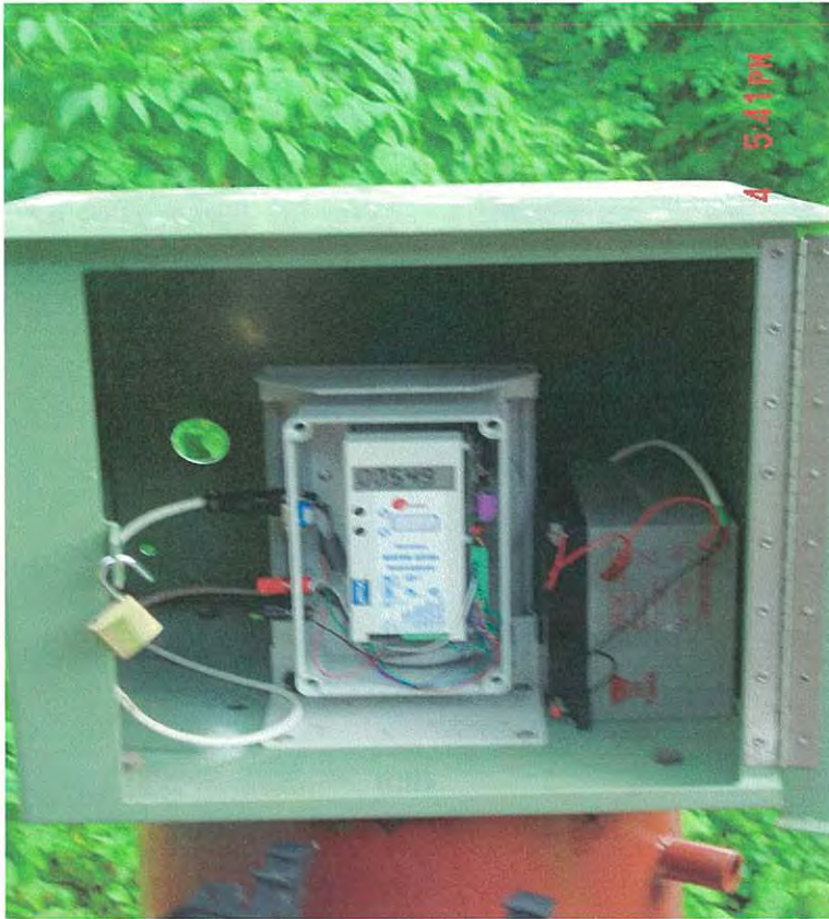
Fanafo Hydrologger and batterie to record waterlevel and rain fall. (Working)
