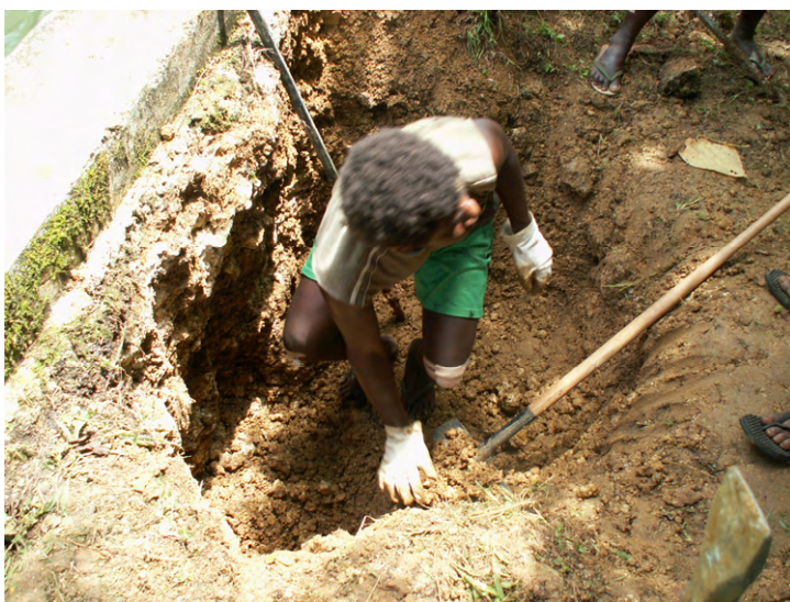
The temporary civil work t has been conducted at some points since last week (Photo 3).
