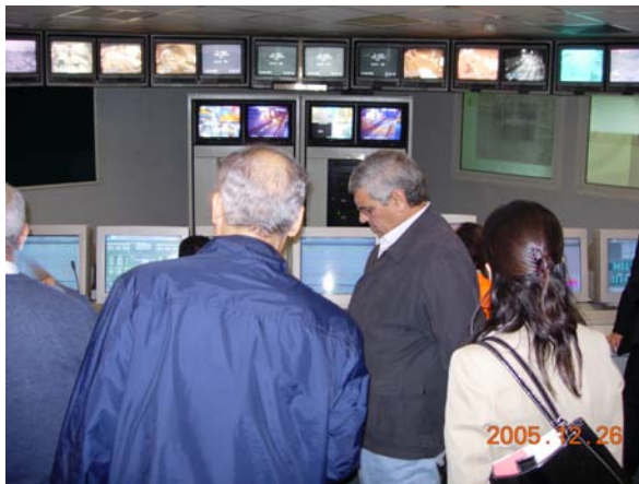
Figure 8.3-3 Traffic Control Center of Al-Azhar Tunnel
