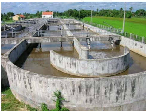
6. Pathumthani STP (After rehabilitation)
