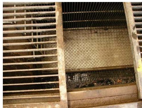
4. Manual raked screen (after improvement)
