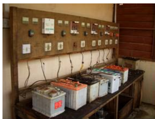
Battery Charging Station system (Wacheu)
