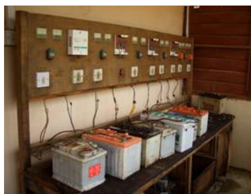
Battery Charging Station system (Wacheu)
