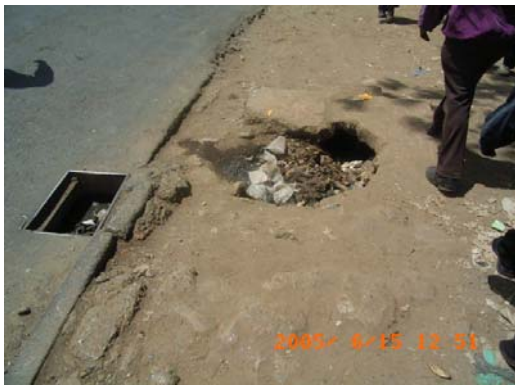
Drainage: Mal-function and poor maintenance
