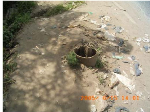
Street Light: Non-functional
