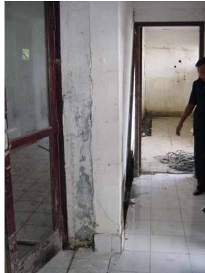
Damage of column
