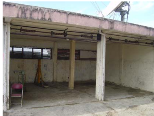
Damage of Garage
