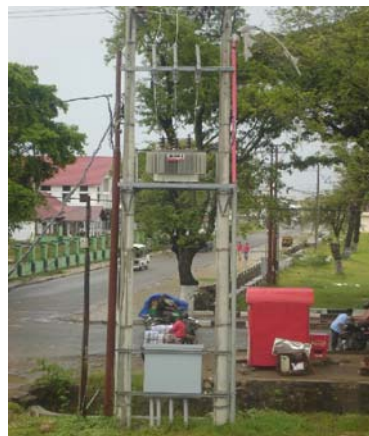
Electrical Pole from PLN
