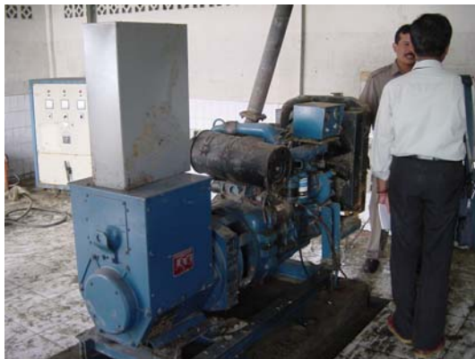
Damage of Generator
