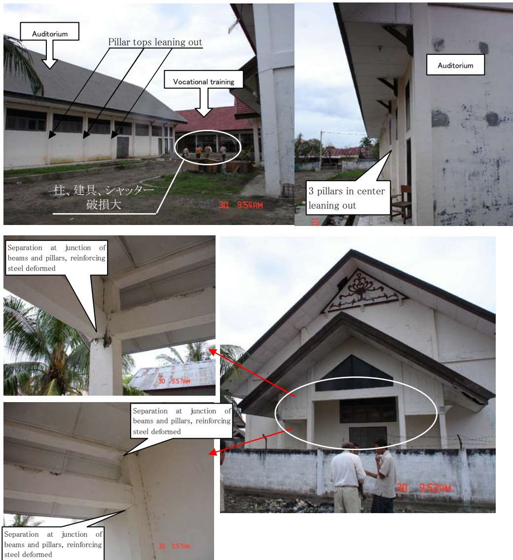
Figure 1.1.10 Damage Condition of Jroh Naguna Orphanage Auditorium
