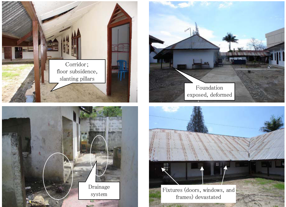
Figure 1.1.9 Damage Condition of Nirjala Orphanage
