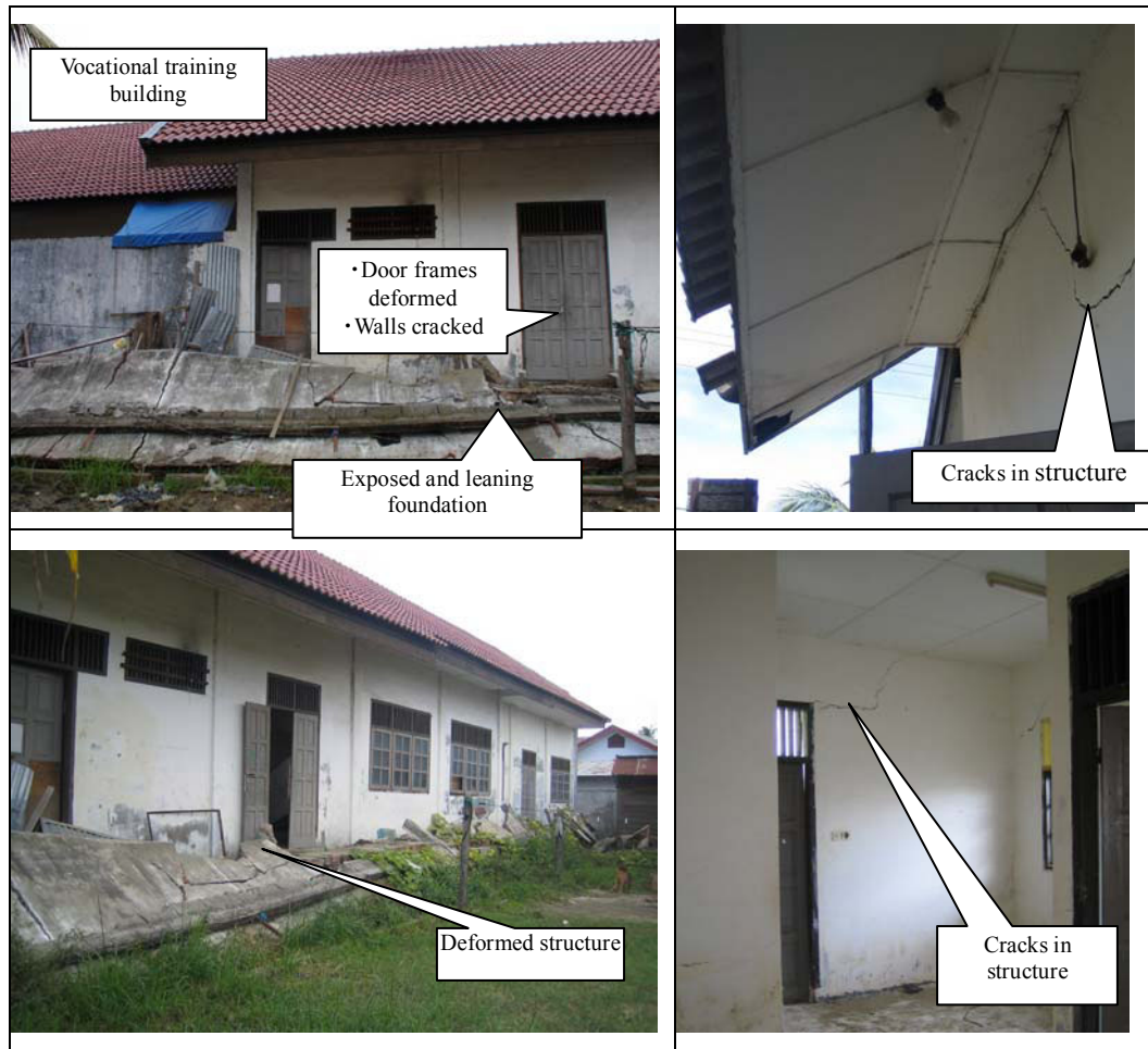
Figure 1.1.11 Damage Condition of Jroh Naguna Orphanage Vocational Training Building
