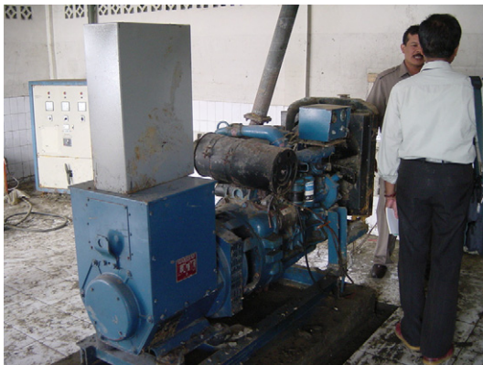
Damage of Generator
