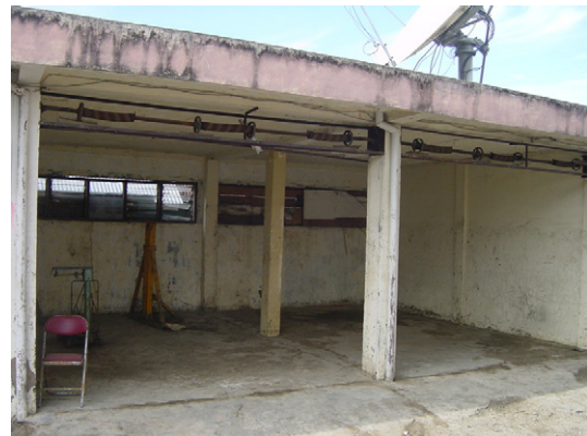
Damage of Garage
