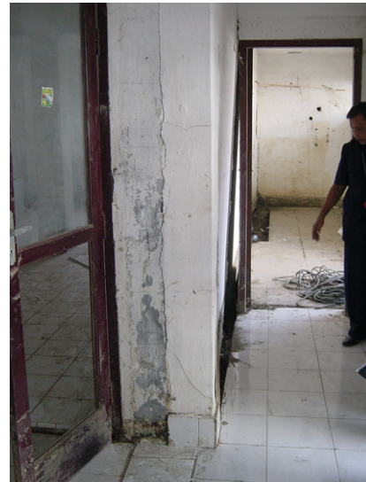
Damage of column
