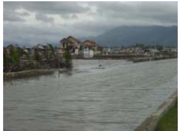
Collapsed River Dike (Doy River)
